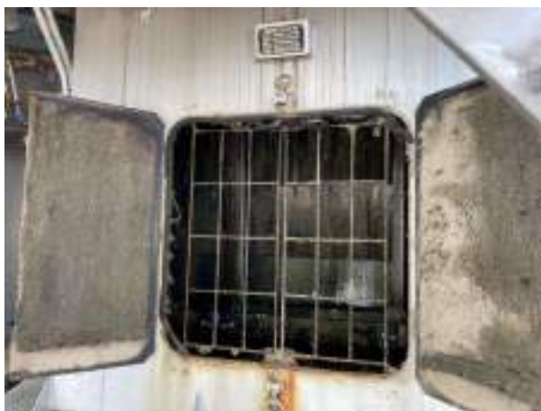
[沈砂掻揚機内部]
